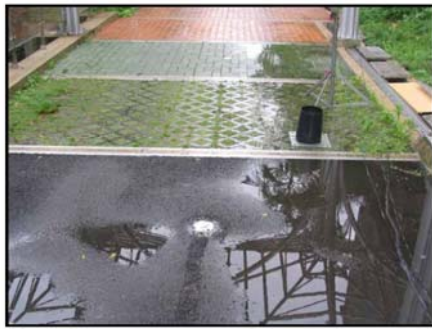
Water accumulation after rainfall
